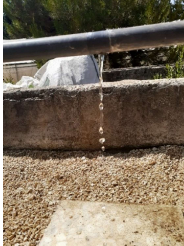
Photo 4.2: UASB effluent to constructed wetland. Date: 06.08.2019
