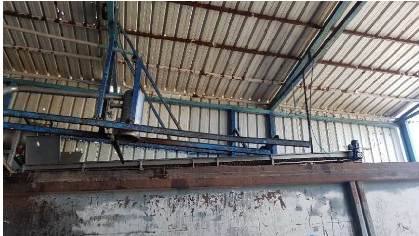
Photo A-1 and 2: Poultry Slaughterhouse feather separation system
